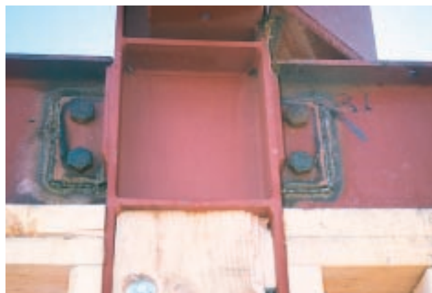
Figure 4. Steel I-beams can be prepunched for bolts; with tube steel, it's easiest to fasten lumber with powder-actuated fasteners.
