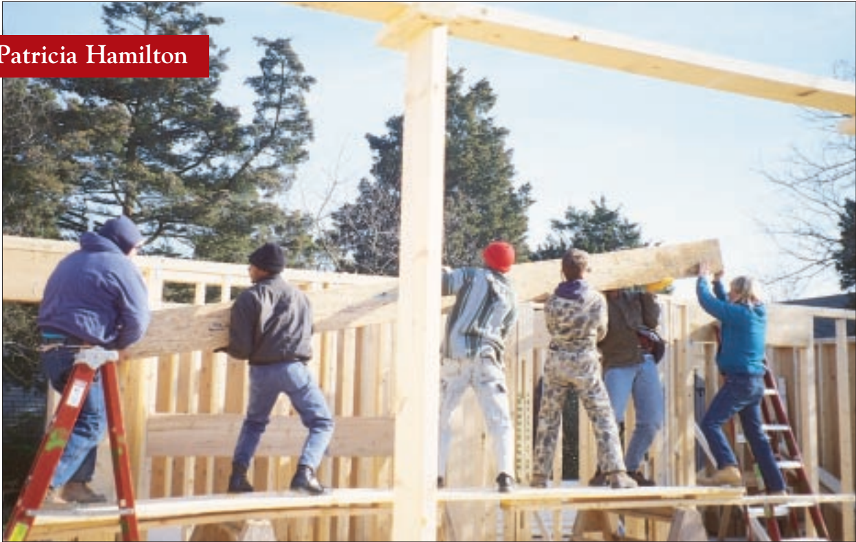
A Parallam beam is heavier than an equivalent-strength steel I-beam. The author's crew lifts beams up to 16 feet by hand; beyond that, they use a crane.
