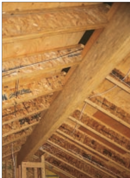
For a ridge beam, the author saves time by using a single piece of Parallam rather than laminating a multiple-member LVL beam.
